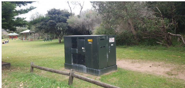
Gov Phillip Park (western side) substation
